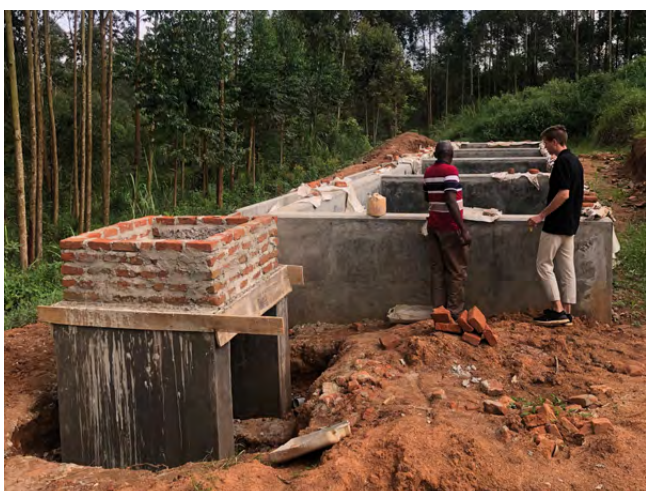
Construction of a faecal sludge plant in Fort Portal, Uganda. ©Elke de Buhr/SHF
